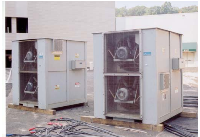
Two 2500kW Load Banks Testing Diesel Generators At Casino
